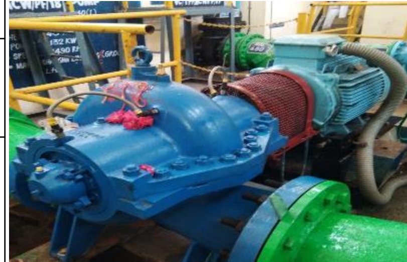
Energy Efficient Pump with 45KW motor in place 132KW
