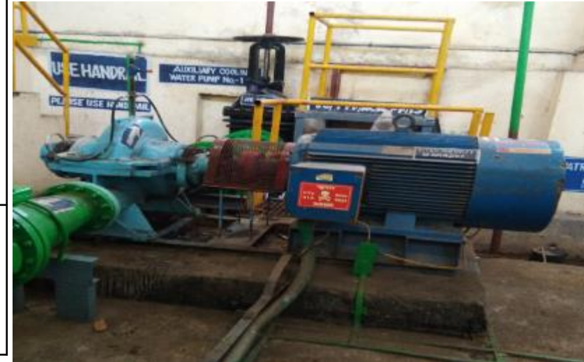
Before- Pump with 132KW Motor
